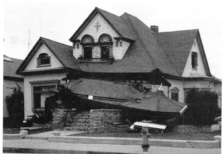
The Jensen House as it looked after the October 17th earthquake. Photo by Kay Peterson.
